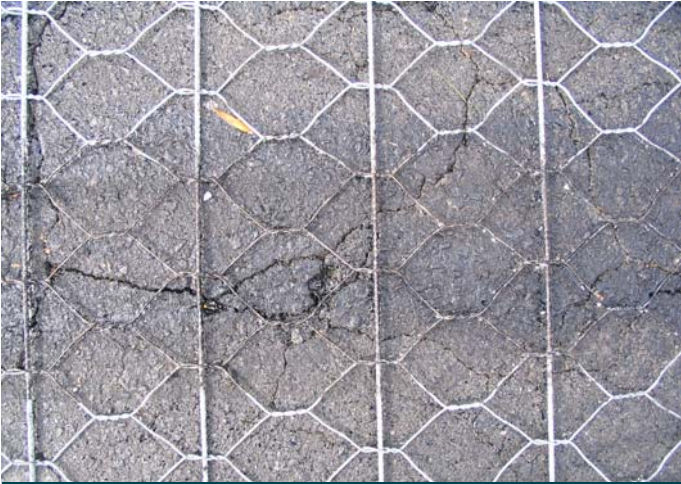
Detail of crack beneath Road Mesh™
