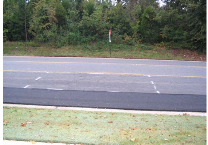
Existing fatigued area
