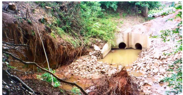
Severe erosion looking upstream towards outfall
