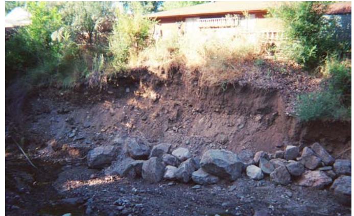
The eroded river bank showing debris carried by storm flow
