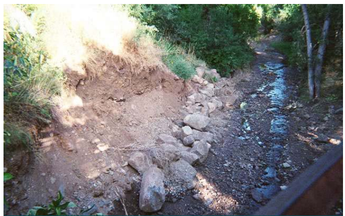
Tucker Gulch after the 1:100 year storm event looking upstream
