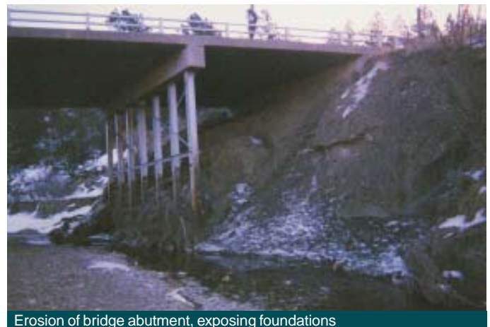
Erosion of bridge abutment, exposing foundations
