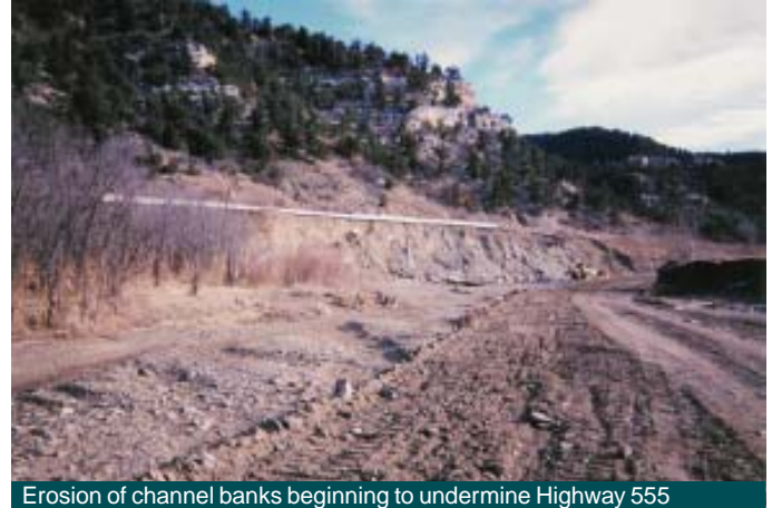
Erosion of channel banks beginning to undermine Highway 555
