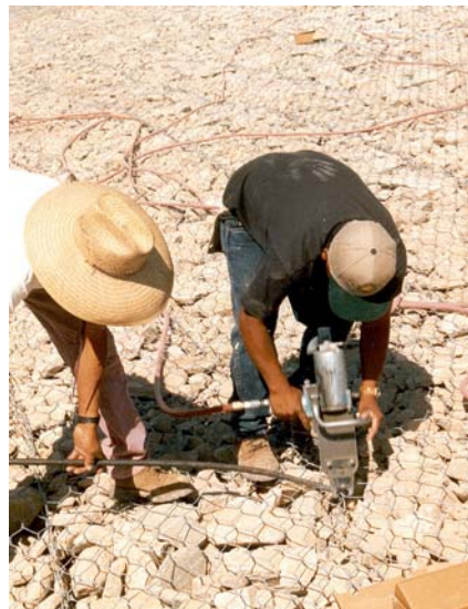
Overfilling and stretching of Reno mattress lids (different project)
