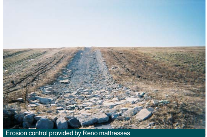
Erosion control provided by Reno mattresses
