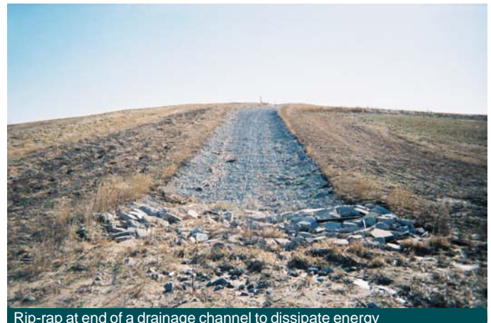
Rip-rap at end of a drainage channel to dissipate energy
